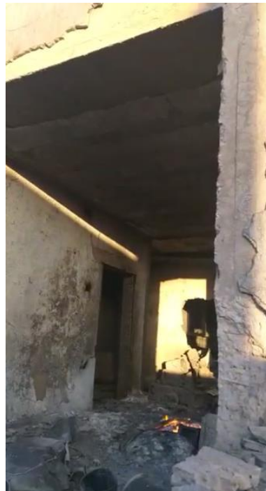
Image 16.3 Damaged infrastructure with characteristics of high explosives damage
