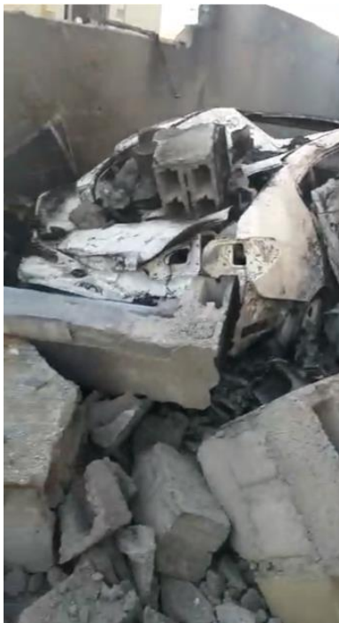
Image 16.2 Damaged infrastructure with characteristics of high explosives damage
