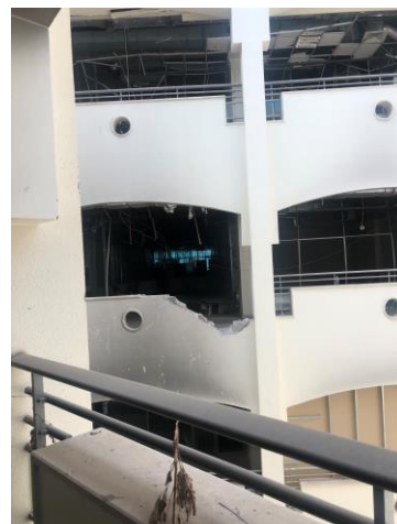
Figure 9.4 Condition of the premises in September 2019
